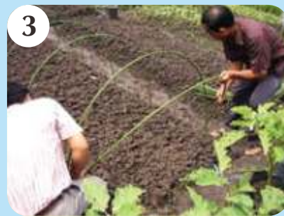
3 At the end of seedbed tunnel pipe is installed with tilting angle of 22°
