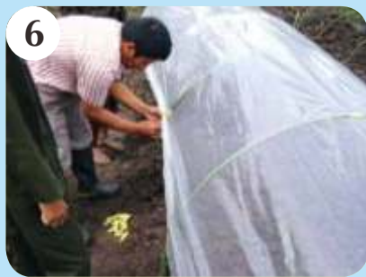
6 Spread the plastic cover on tunnel pipe then clip it with the packer
